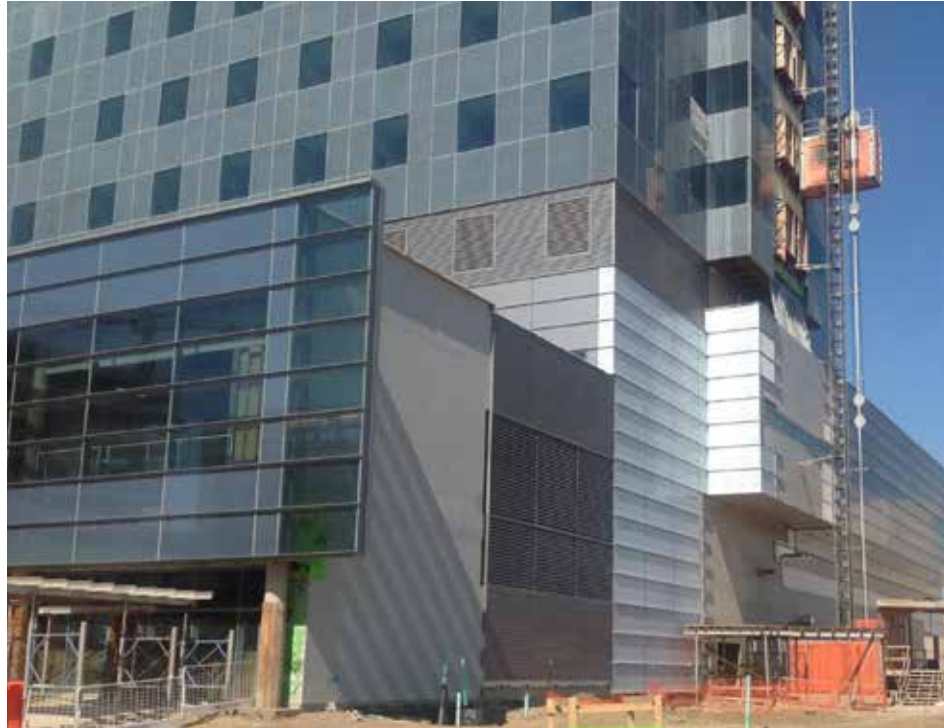
Providing continuity throughout the building envelope layers of protection is imperative for control of air and moisture infiltration.
