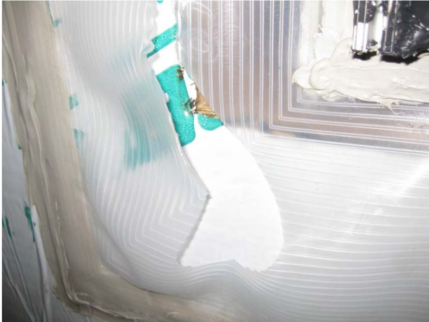
Photo No. 5 Failure of Membrane During -175 psf Structural Load
