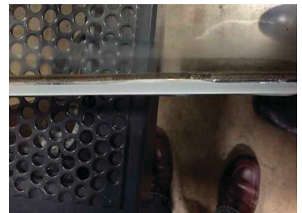
Sealant blow by
