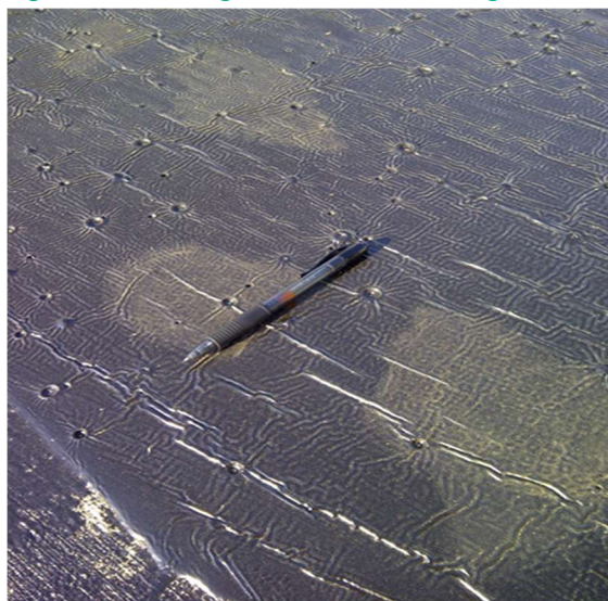
Figure 4 - Pinholing in a membrane during cure
