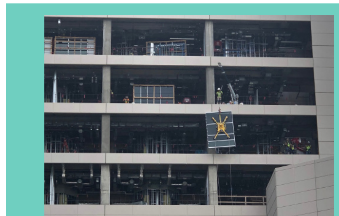
Prefabrication of the ribbon windows expedited this project, as completed window systems were manufactured in a plant and then craned into place.
