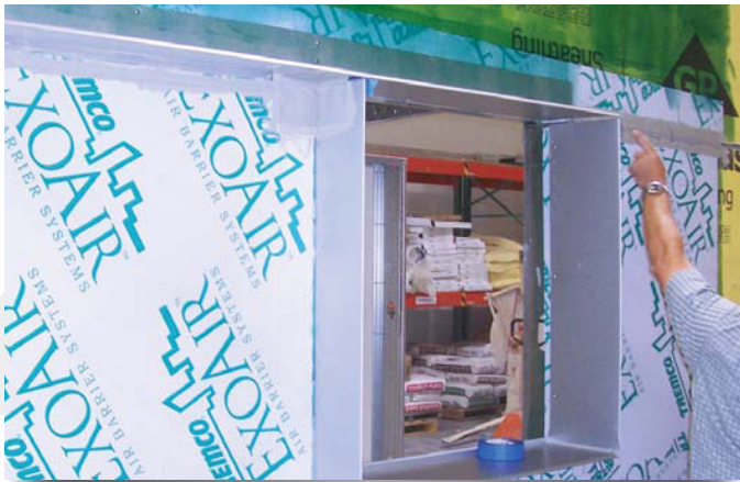
▲ A 30 ft tall mockup was built and submitted to a series of ten tests to determine air leakage under dynamic pressure conditions, ability to withstand structural wind loads, racking and wind-driven rain.
