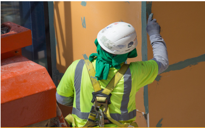
Panels with the air barrier already applied cuts out a step on the installation process.
