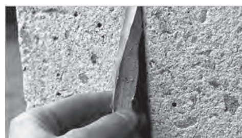
FIGURE 3.6b – SEALANT ADHESIVE BOND LOSS
