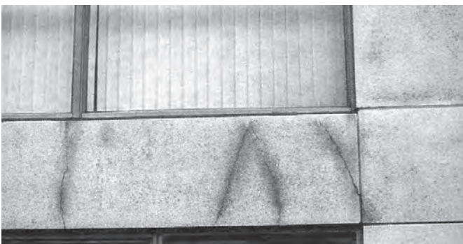
FIGURE 3.1 – WALL CRACKING PATTERNS
