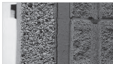
FIGURE 3.6a – SEALANT ADHESIVE BOND LOSS
